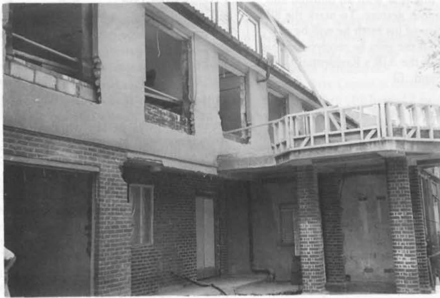
A new roof garden is under construction for the benefit of residents at Osmond House in The Bishop's Avenue.
